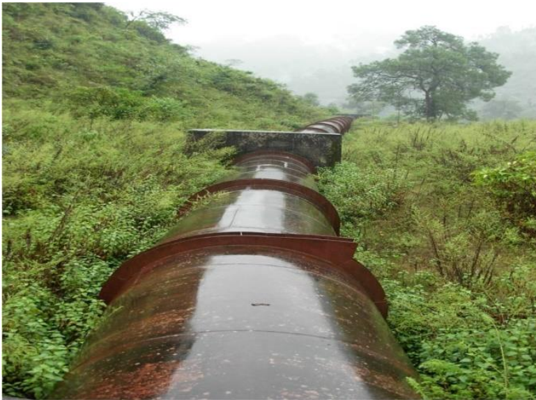
Figure 2 Penstock of Rajwakti SHP
