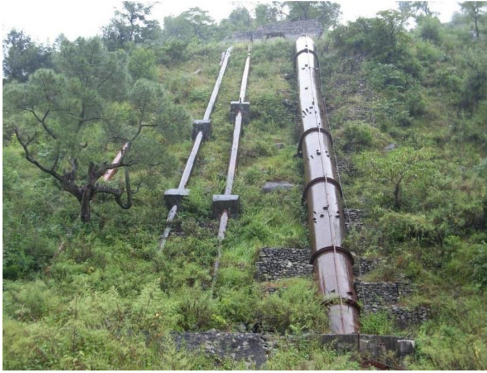
Figure 3 Surge tank pipe of Rajwakti SHP
